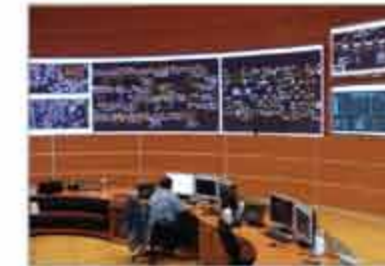
UTILITY CONTROL ROOM Mexico 8 × 4
